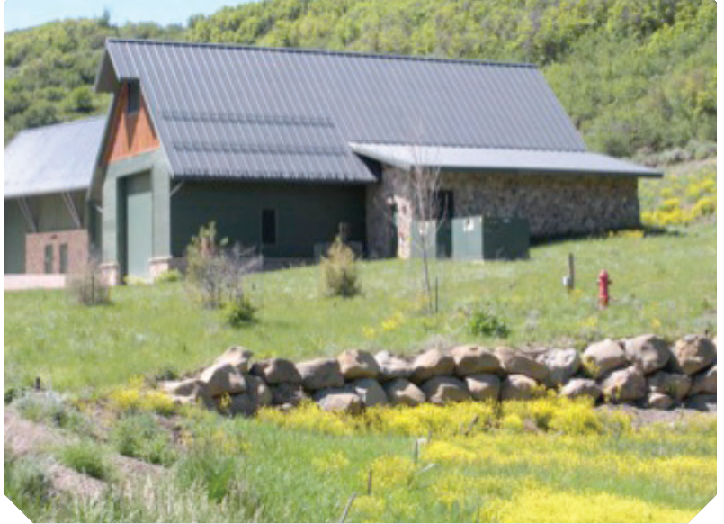
The GIS substation was nestled into the hillside with site restoration in progress.
