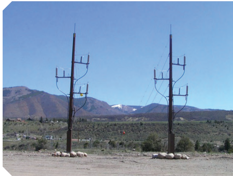
These towers bring the 115 kv line across the Roaring Fork River where it goes immediately under ground to begin its seven-mile journey under Highway 82 to the GIS substation.
